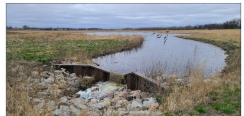
An outlet structure was installed as part of a wetland restoration on this MN CREP easement in Freebourn County. Restoring the wetland reduced pressure on the county ditch system while providing water storage and wildlife habitat. Photo Credit: BWSR
