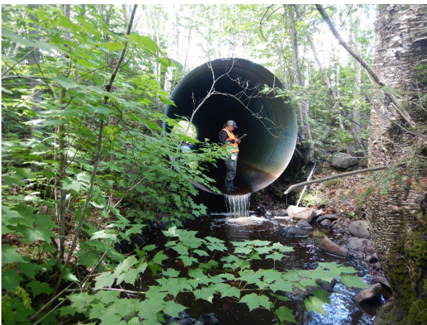
Figure 1. A perched culvert on the mainstem of Irish Creek. Photo Credit: Cook County SWCD.
