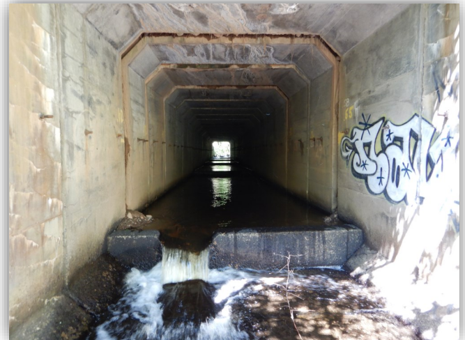
Above: The culvert interior and the barrier in place that prohibits fish passage and degrades fish habitat.
