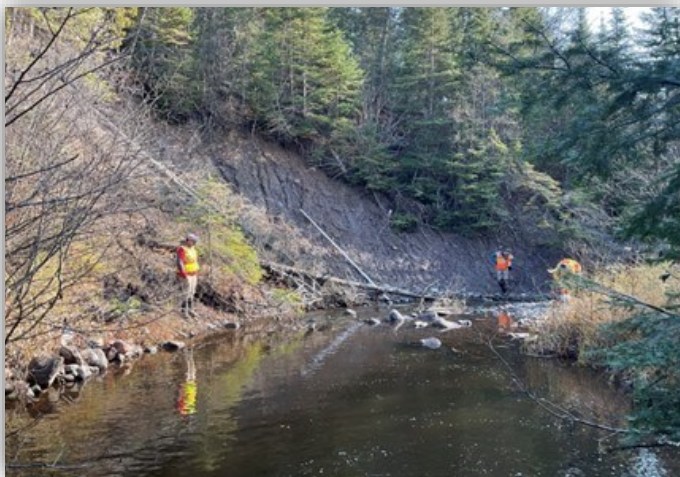
Above: Downstream view at the culvert outlet and an example of the bank erosion caused by increased river velocities due to the improperly sized culvert.
